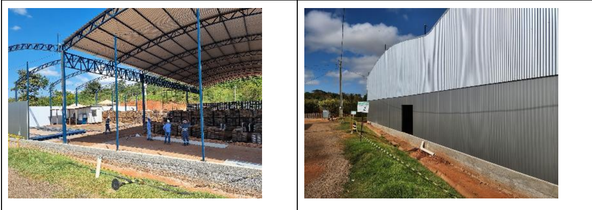
Figure 12.4 Core Shed installation during 1 st visit, and after complete construction on 2 nd visit
